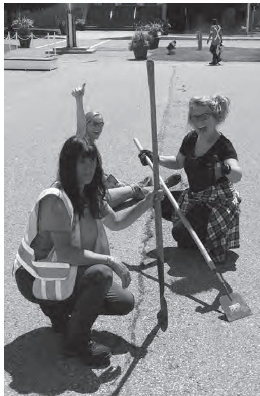
Construction Engineers (CE) Roads and Grounds crew prepared the parade square for the Change of Command (CoC) parade on Aug. 11. CE civilian employees are delighted to contribute to the success of the CoC parade. Photo submitted by Sgt. Steven Duplisea
