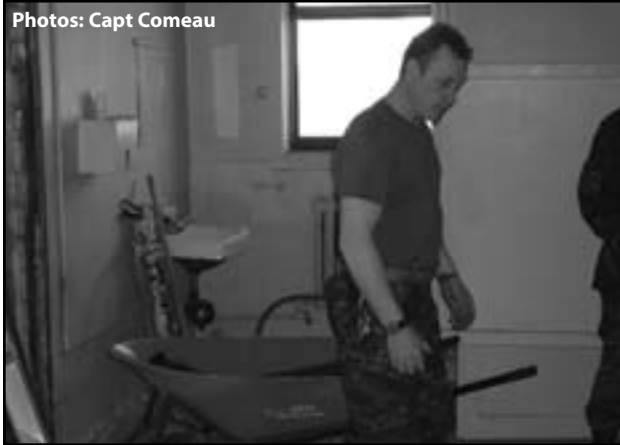
Photos: Capt Comeau 81 AEF personnel hard at work renovating the Heavy Equipment washroom.
