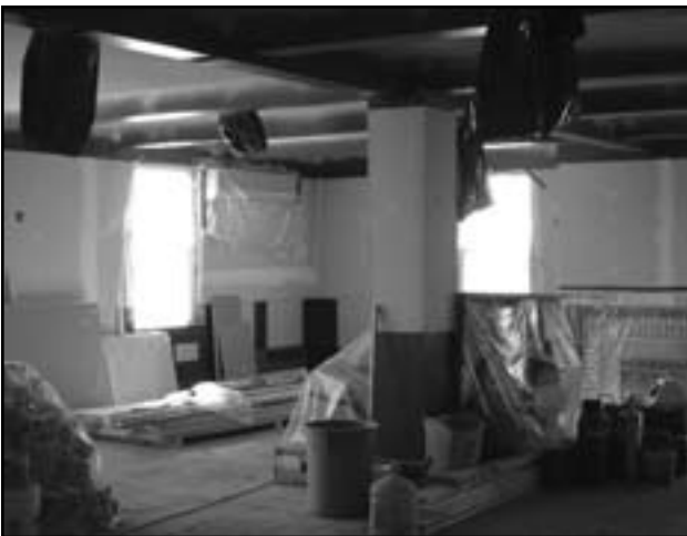
An interior shot of the renovations at the WO's & Sgts' Mess on the south side.
