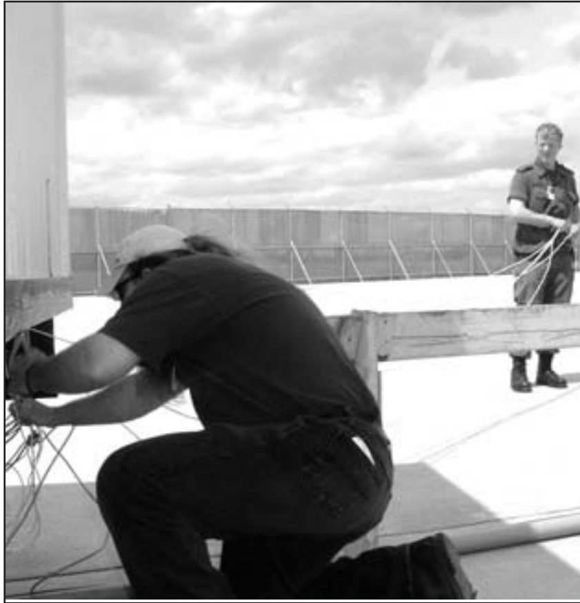
WTISS Linemen, Mr Neild and Pte Turpin are installing communication cables in the 424 Sqn trailers. 424 Sqn moved into the trailers while the the 9 hanger extension renovations are underway.
